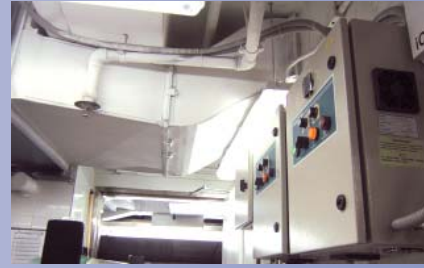
Exhaust Vent Duct
